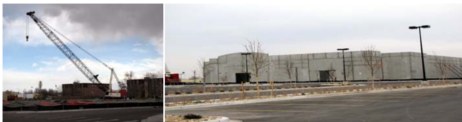
Pictured: On the left, the Sprouts site on Monday; on the right, the walls at Sprouts are already up. Sprouts will open in October 2009 at The Gardens on Havana
